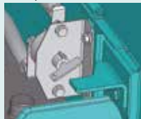
Battery disconnect switch
