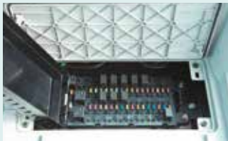
Easy-access fuse box.
