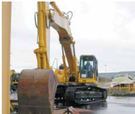
High reach demolition machine, digging boom installed, with simultaneous twist and bend loading.
