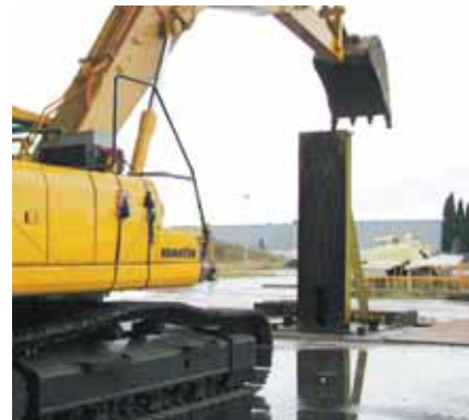
High reach demolition machine, twisting load applied to new demolition first boom.
