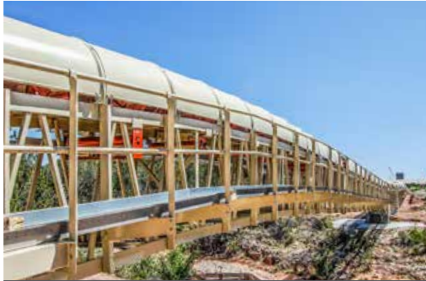
TRUSS FRAME CONVEYOR
