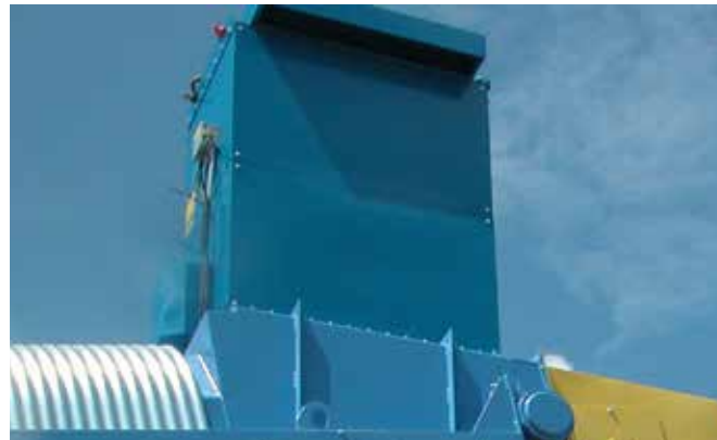
DUST COLLECTION SYSTEM
