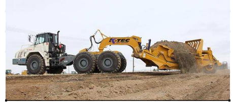
Sand + Clay / Colorado, USA
