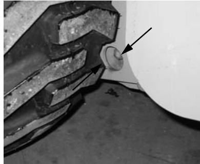
Figure 38 Remote Engine Oil Drain
